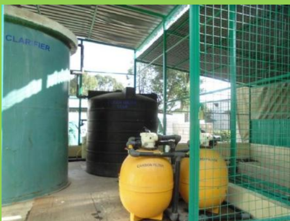
PFIL's Effluent Treatment Plant
